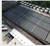
Carlsberg Britvic Brewery- Cambridge Flat Roofing Company Ltd, working with Garland UK
