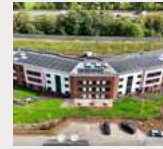
Seabrook Orchards- NRA Roofing & Flooring Services Ltd, working with ICB (Waterproofing) Ltd
